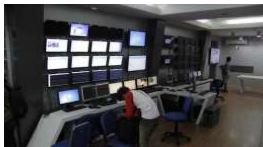
Figure 18. Interior of TIC Monitoring (Interconnection) Room (Source: Data Personal )
