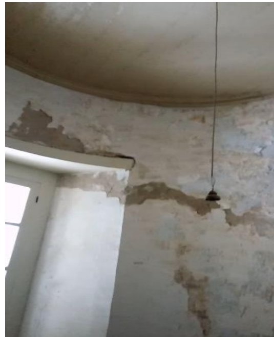
Figure 6. Damage on the inner wall
