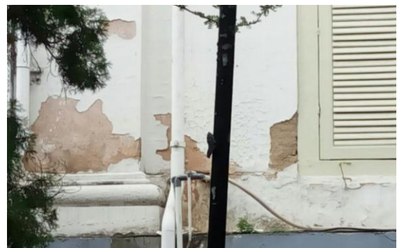
Figure 7. Damage on the outer wall surface
