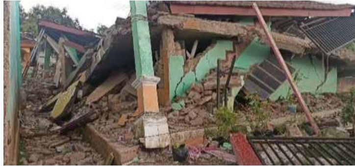
Figure 9. Foundation Structure Failure in Supporting Axial and Vertical Loads
