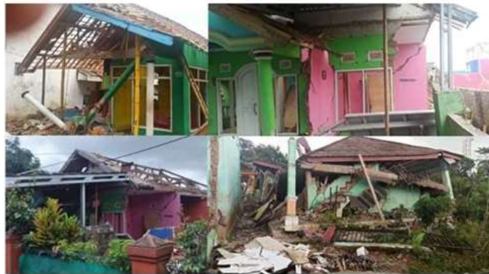
Figure 5. Column Structure Failure Unable to Support Beam and Roof Framework
