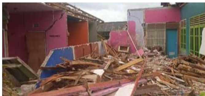
Figure 6. Beam Structure Failure Due to Poor Design for Load Bearing
