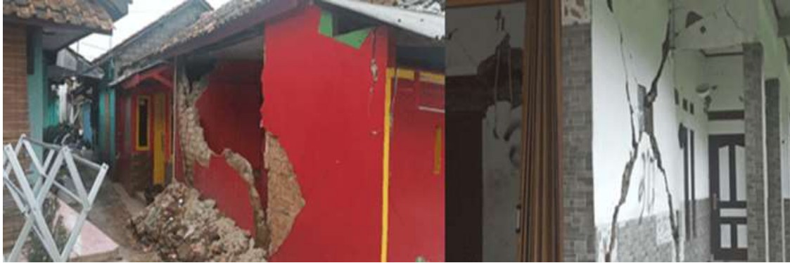
Figure 7. Photo of Wall Collapse Due to Poor Design and Lack of Anchors/Reinforcement in the Columns to Bind the Wall
