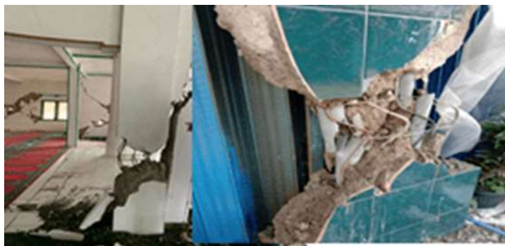
Figure 10. Failure in Rebar Hook Installation in Columns
