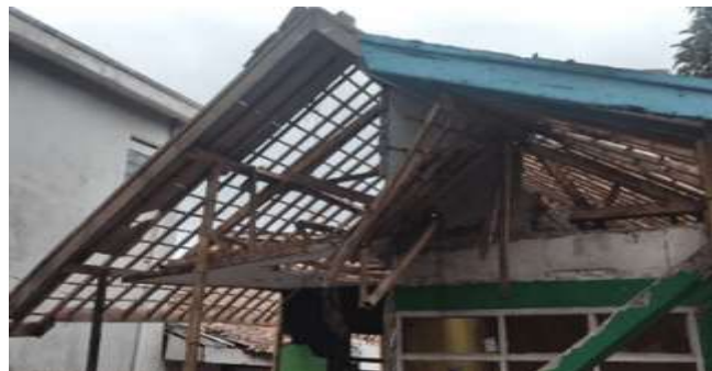
Figure 8. Failure of Connections in the Wooden Roof Frame
