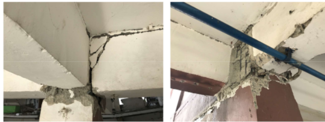
FIGURE 8. Damage of beam-column joint due to earthquake
