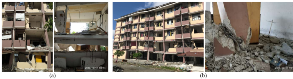
FIGURE 1. Pictures of damaged rental low-cost housing flat Lere: (a) major architectural damage, (b) major structural damage concentrated on base columns undergone compression failure and combined shear and tensile failure
