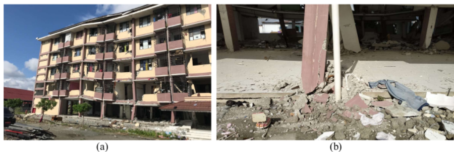
FIGURE 5. Structural damage: (a) compression failure in column, (b) tensile-shear failure in column
