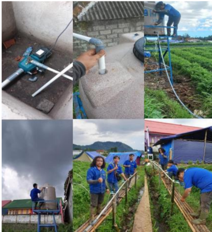
Figure 2. Clean Water is Ready for Access in Cibeureum Village, Cugenang, Cianjur
